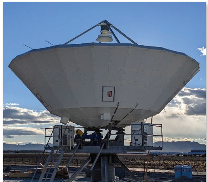
A Kratos antenna installed with proprietary subreflector tracking technology. Photo Credit: Kratos
